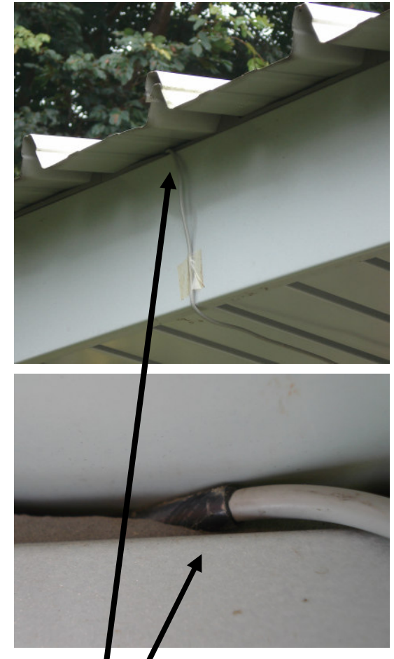
Sensor to measure roof temperature
